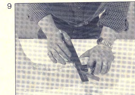
Three supports are clamped together and marked for location of slats. Note that supports are slightly flattened for easier attachment of slats.
