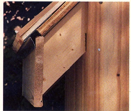
THE INNER RAFTERS are notched where they pass through the wall boards. Note metal drip edge between sheathing and fascia
